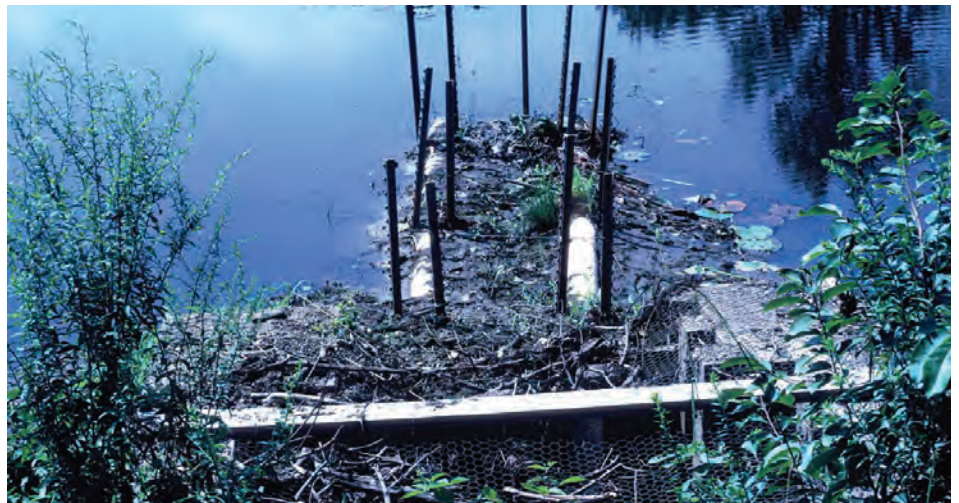
Knowles 2 Pond control structure showing damming at overflow area and around PVC piping, but water level remaining level due to underwater drainage in pipes, 1989.
