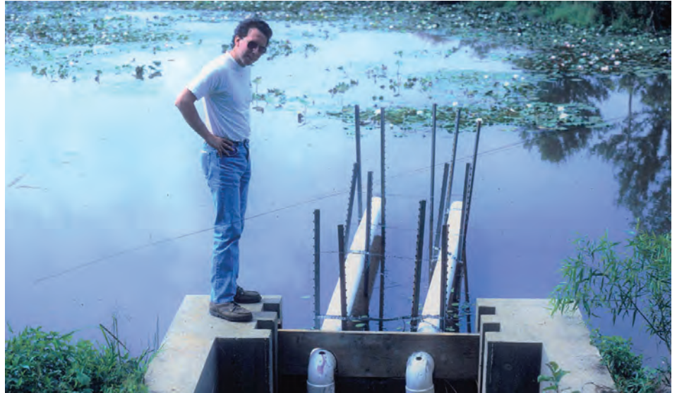
PVC piping to maintain constant water level at Knowles 2 Pond control structure. Inspected by Friend of Patuxent, Kirk Wineland, 1987.
