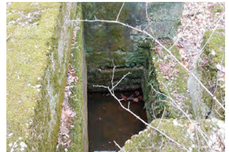
Opening view from top showing mill area where a wooden water wheel might have existed.
