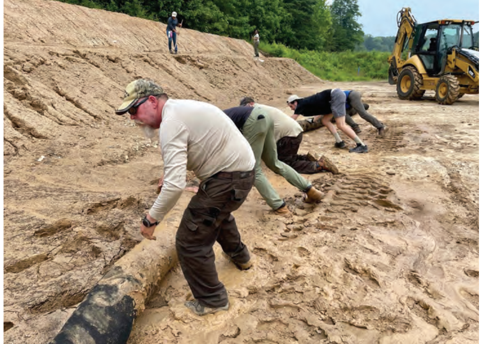
Youth Conservation Corps and Career Discovery interns, along with staff from Patuxent and other refuges in the region, worked together to stabilize the berms at the firing ranges following removal of 126,000 tons of lead from the soil.
