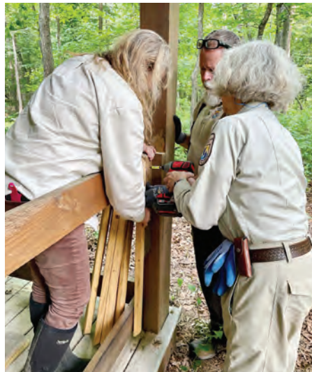
Refuge staff (Biologist Sandy Spencer, Facility Manager Martin Brockman, Ranger Diana Ogilvie) worked together to complete renovations of the Dr. Chandler S. Robbins Outdoor Education Center, work initiated earlier this summer by Union Sportsmen's Alliance volunteers.
