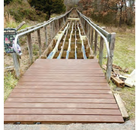
Much-needed renovation of the Lake Redington boardwalk is underway, complete with composite decking.
