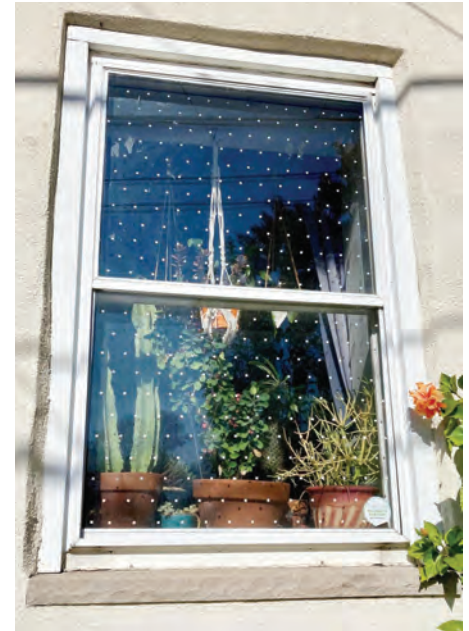
Residential window with bird-safe window bird collision deterrents applied.
